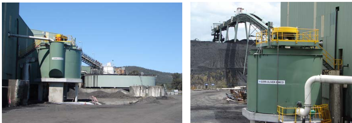
WEMCO 130m 3 Smart Cell at Stratford Coal
