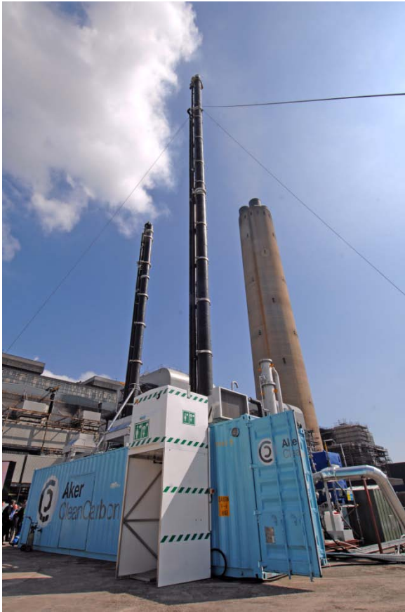
Mobile Test Unit, Longannet Power Station
